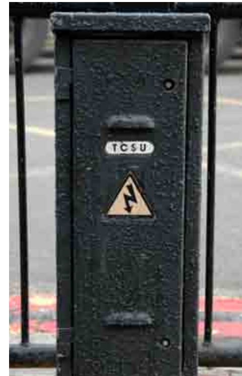
Utility Cabinet with anti-graffiti coating Tottenham High Road
