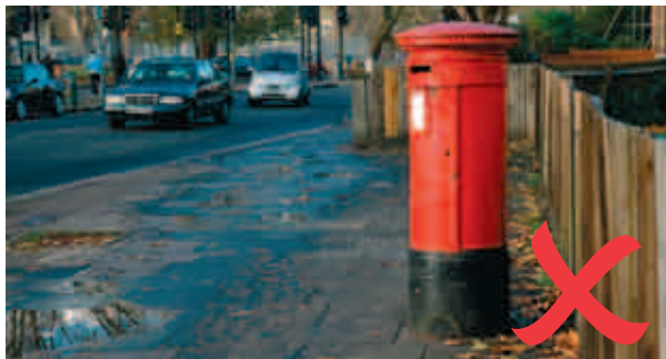
Bad practice - poorly laid materials can result in puddling.
