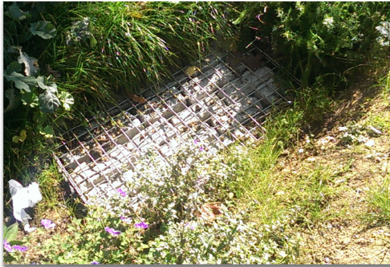
Example of rain garden outlet designed to protect flow control from blockage
