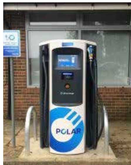
Figure 3. Rapid (43 kW) charging point
