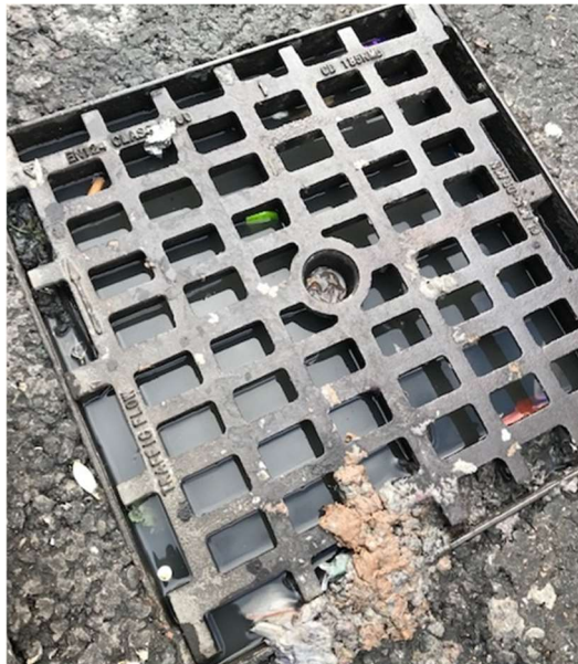
Figure 5-4 Blocked gully outside 490 High Road, 28th October 2021
