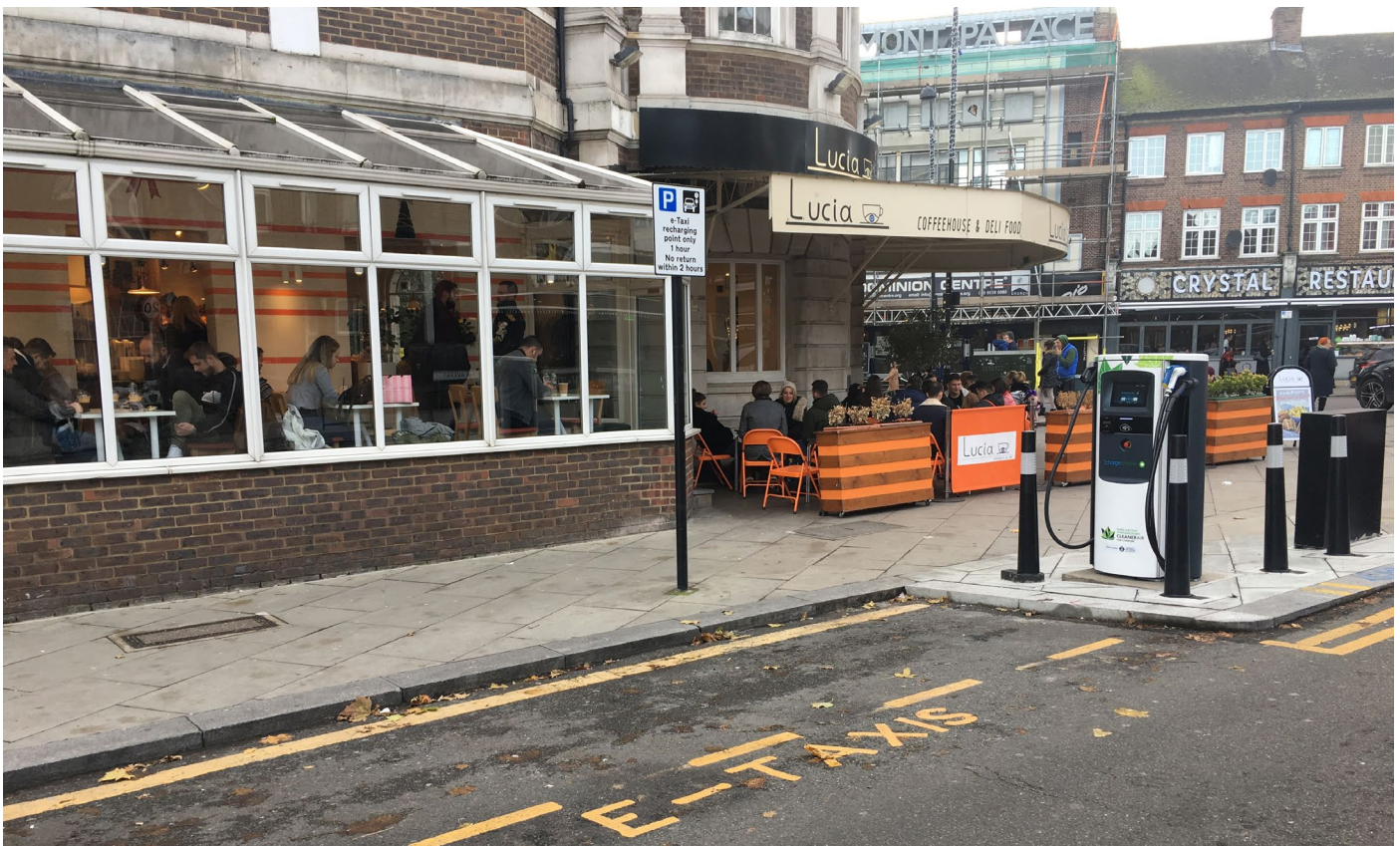
Figure 5. Rapid charging point on Gladstone Avenue (N22) on a build-out in the carriageway.
