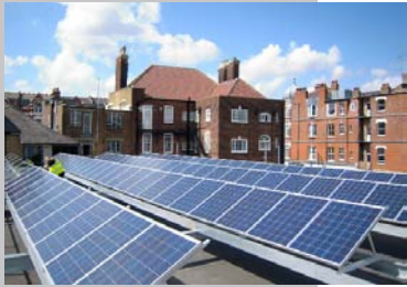
Marks & Spencer PV panels
