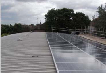
Fortismere solar pv panels
