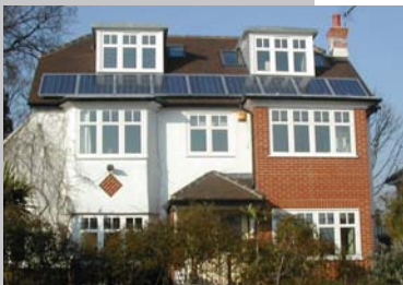
Springfield Avenue PV
