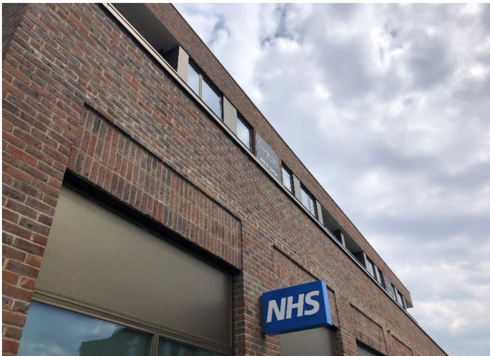
Image: Clarion Housing Group (Latimer) Evergreen, Green Lanes – 133 apartments and duplexes and new health centre.
